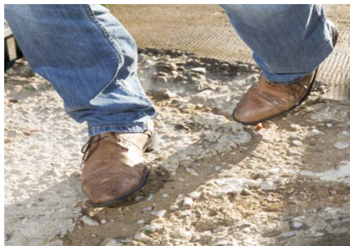
Before: potholes on the bridge
