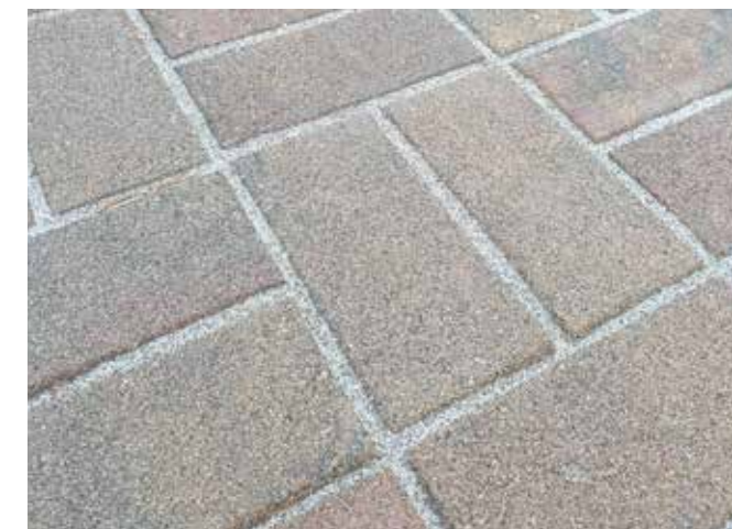
ROMPOX® - FUGENSAND NP + D7000 Joint Strengthener & Surface Sealer installed on a concrete interlocking patio
